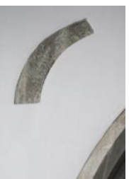
Stone segments of the earliest windows of the church can be seen above the arch in the wall between the chancel and the Lady Chapel.
